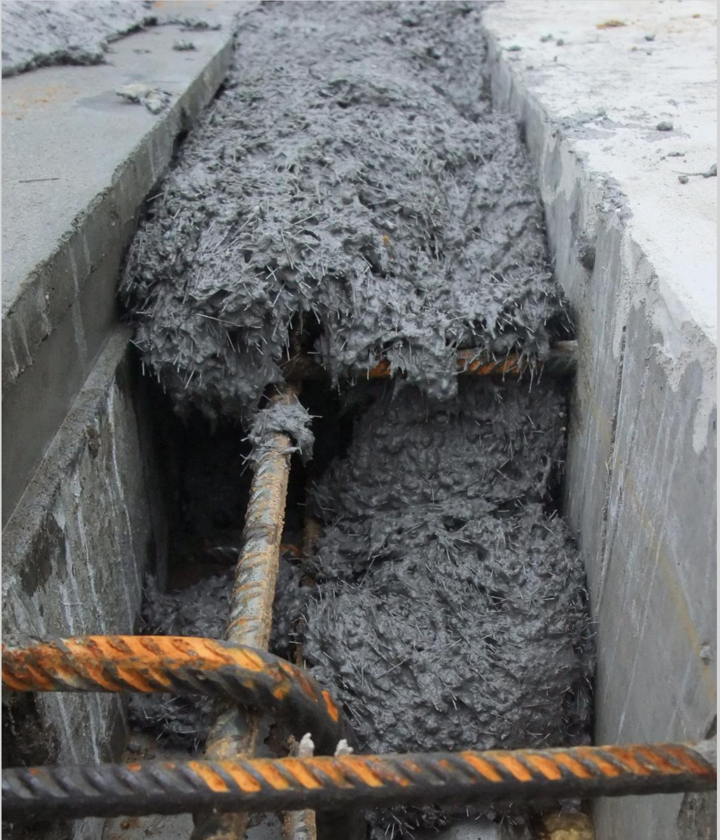
Figure 8.28: Close up picture of the high strength steel fibre reinforced concrete (JointCast).
