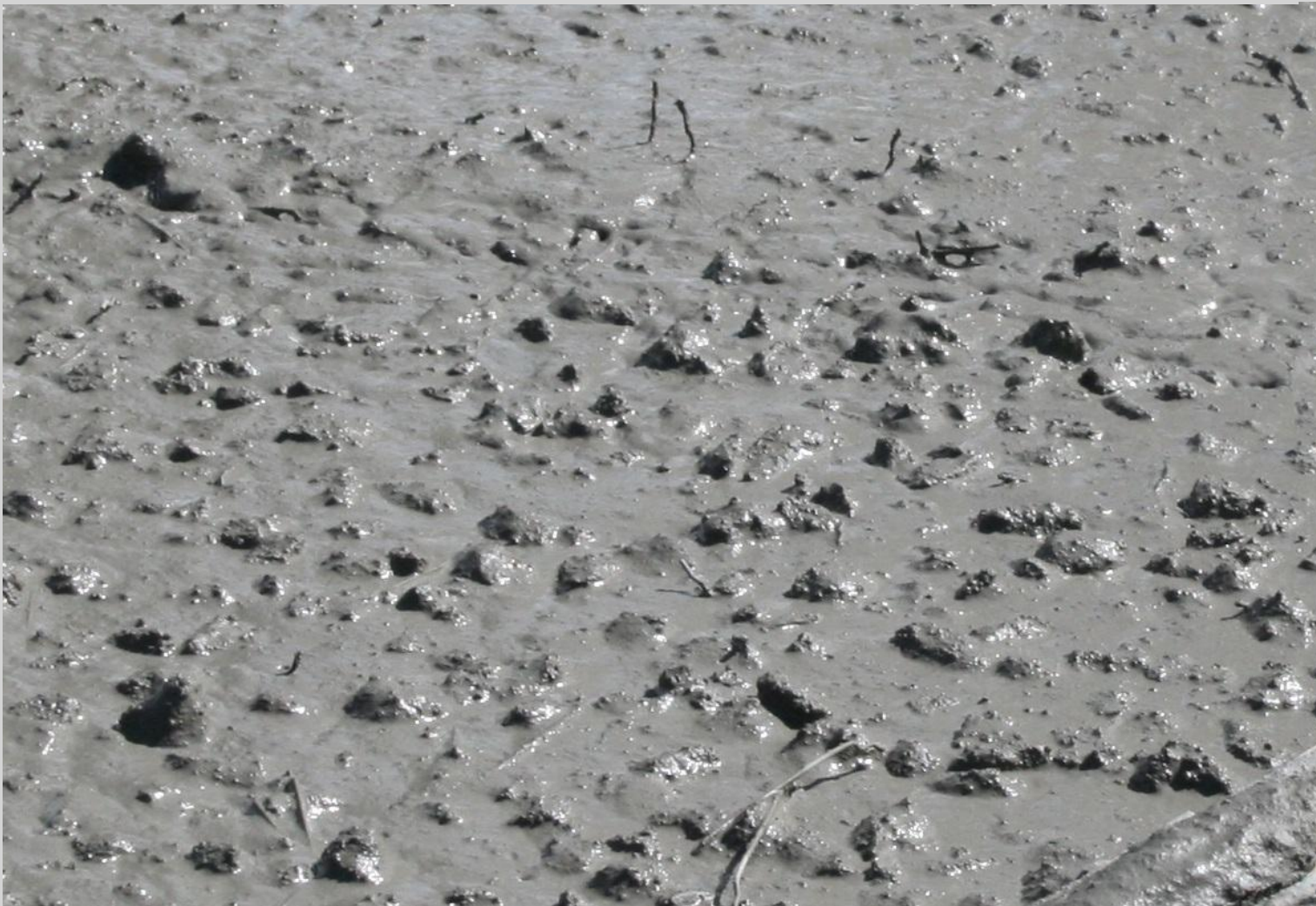
Figure 8.6: Typical surface of SFRSCC just after casting and before any surface finish procedure has been applied.
