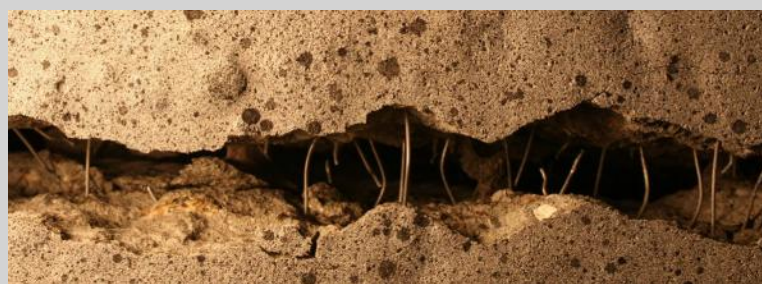
Figure 1.1: Top: Casting of conventional vibrated concrete. Bottom: Cracked section of steel fibre reinforced concrete.
