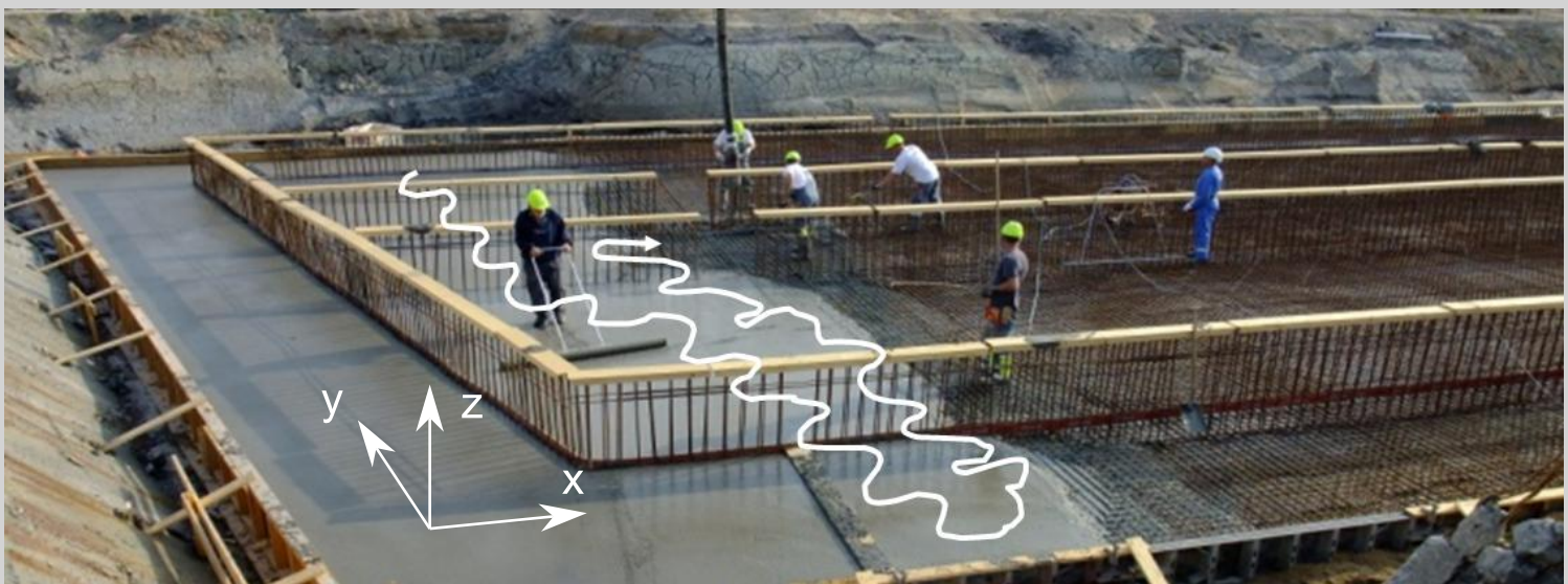
Figure 7.60: Illustration of the casting procedure applied for casting of the foundation slab.
