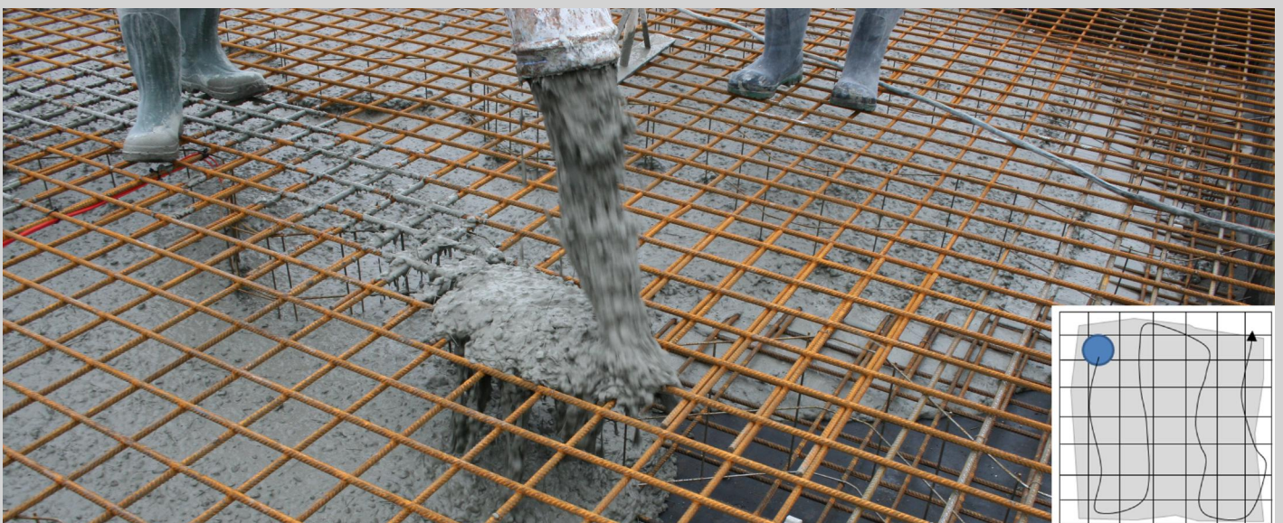
Figure 8.4: Fibre accumulates on the top reinforcement mesh when the pump hose is not moving (top). Fibres do not accumulate on the top reinforcement when the pump hose is moving (bottom).
