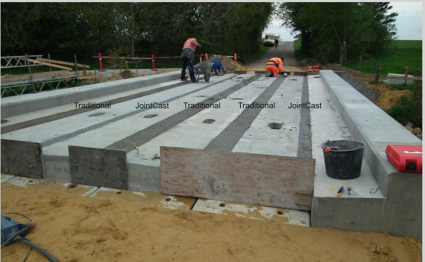
Figure 8.29: Top: Vibration of the traditional concrete and the high strength steel fibre reinforced concrete. Bottom: Picture after casting and finishing of the joints.
