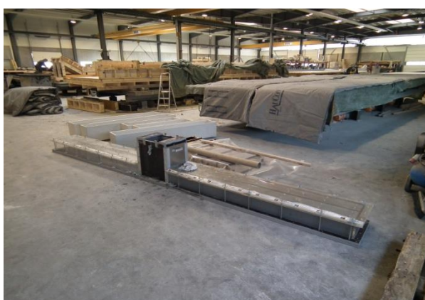
Figure 3: New formworks to produce long 2m beams. See-through acrylic sides make it possible to monitor flow.
