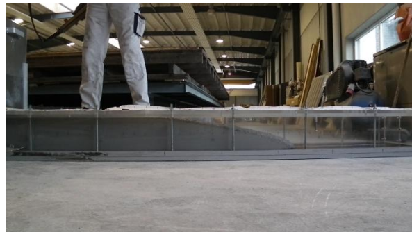
Figure 4: Casting of CRC beams at HiCon facilities. The flat slope of the casting front indicates a high viscous, slow flowing concrete.
